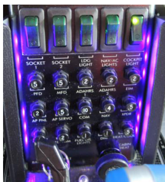
Figure 6 Circuit breakers UV-LED lights
