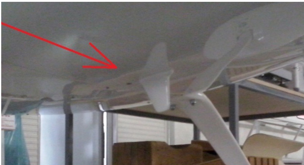
Figure 34-009 XPDR transponder antenna installation
